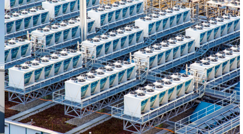
HVAC / Air Conditioning Systems
